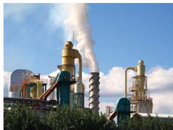
Steam exhaust from power plants
